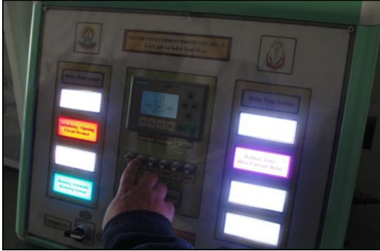
Fig. 10-c. O.C. Protection Unit in operation
