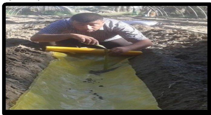
Figure (2) Installation of the SWRT in site as ratio 2:1( width to height).
