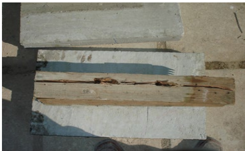
Figure 7: The longitudinal flaw in the timber beam after the failure of the push-out specimen
