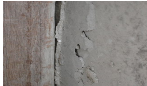
Figure 6: Failure of push-out specimens by crushing of the concrete area surrounding the connector
