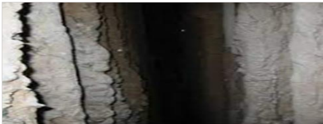
Figure 8: Ash accumulates on the heat exchange tube's inside surface[25]
