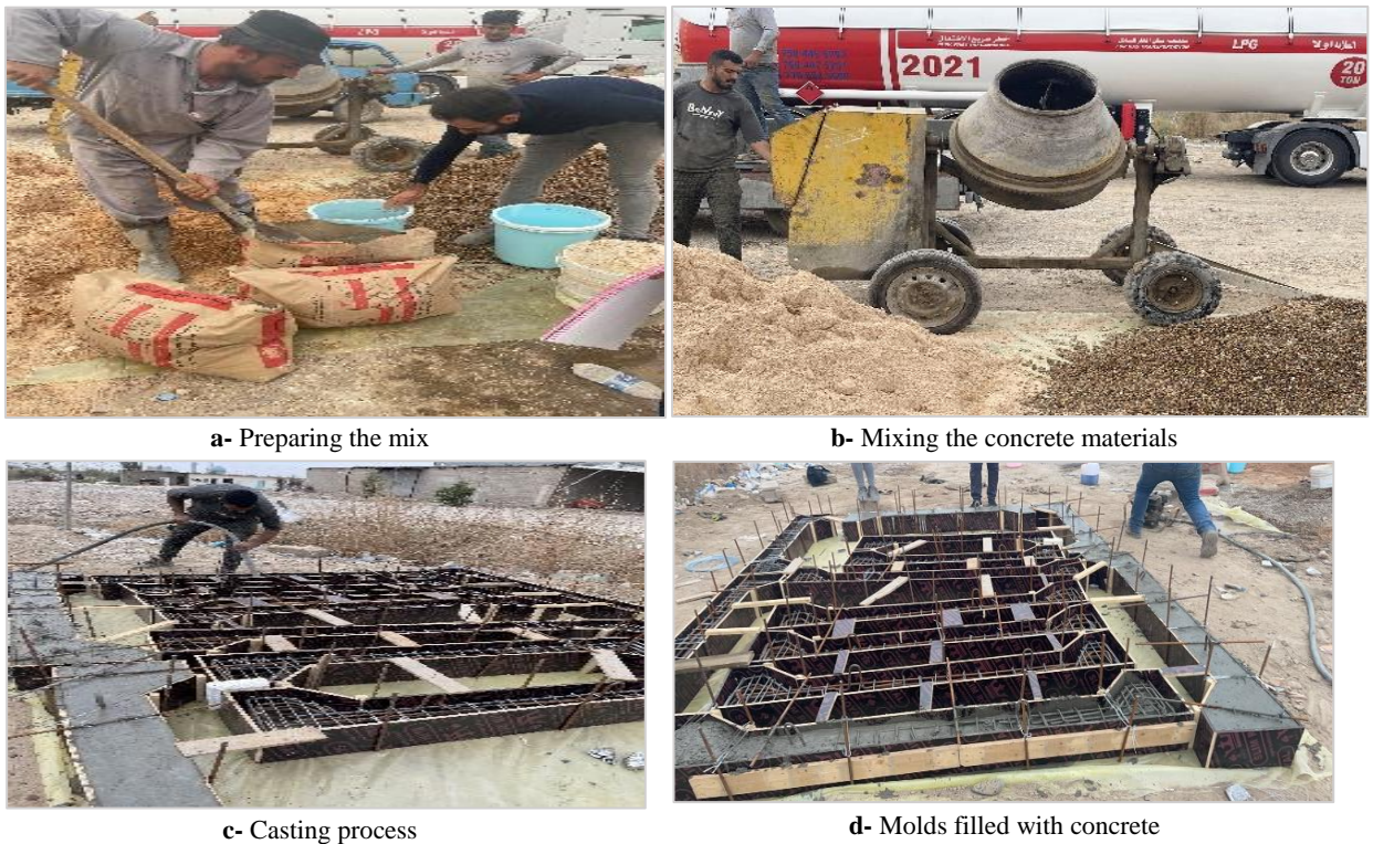
Figure 4: Concrete mixing and casting process, a- Preparing the materials quantity to mixing the concrete to cast test columns, b- Concrete mixing process ,c- Tested columns casting in wood forms, d- Tested columns after casting
