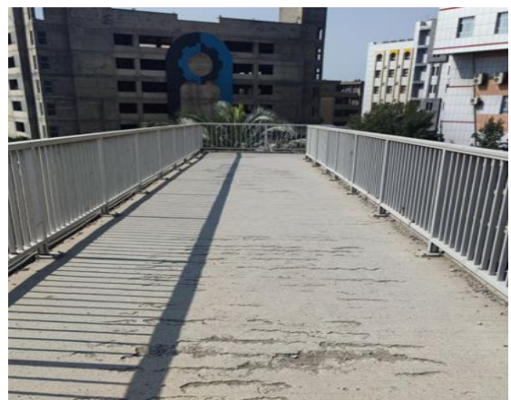
Figure 17: Pedestrian bridges of the University of Technology, worn out floor pavement (Source: Authors).
