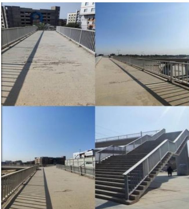
Figure 13. The pedestrian bridge on Muhammad Al-Qasim Road near the University of Technology (Source: Authors).
