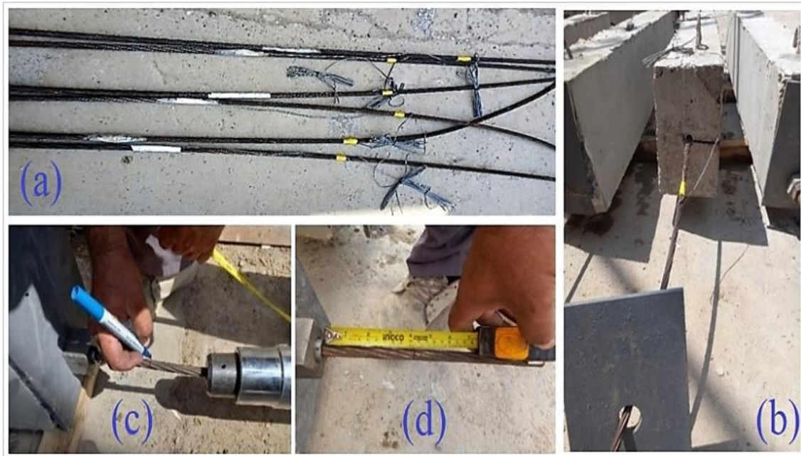
Figure 4: (a)-Fixing a strain gauge sensor in the middle length of strands.(b)- Inserting the steel strand;(c)-Signing a reference point for pulling.(d)-Detecting the magnitude of prestressing the steel strand.
